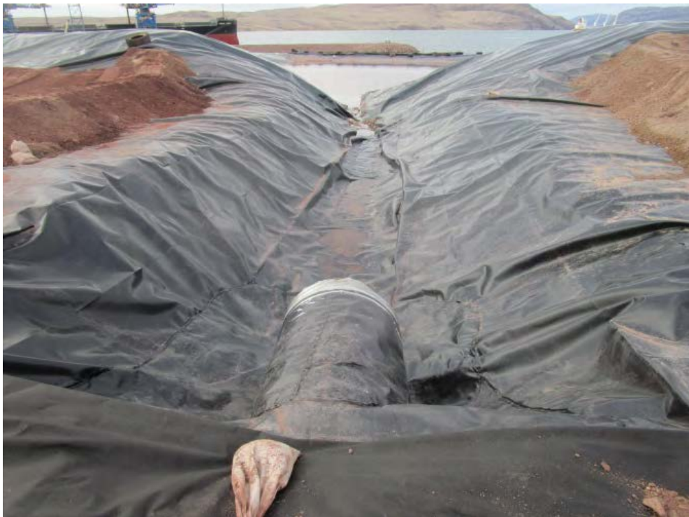
28. Sedimentation Pond East - Liner at south inlet
