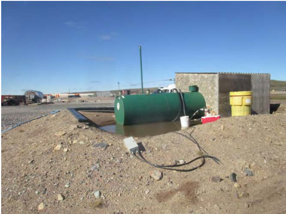
6. Helicopter Fuel Tank Containment
