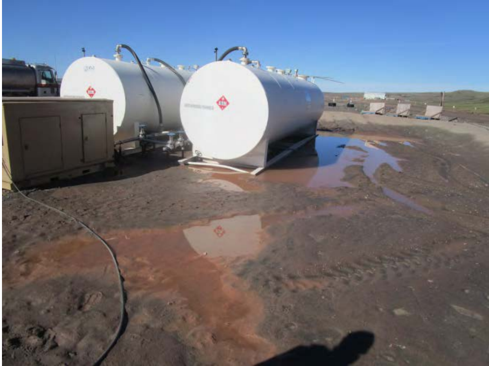
19. Jet A Fuel Containment
