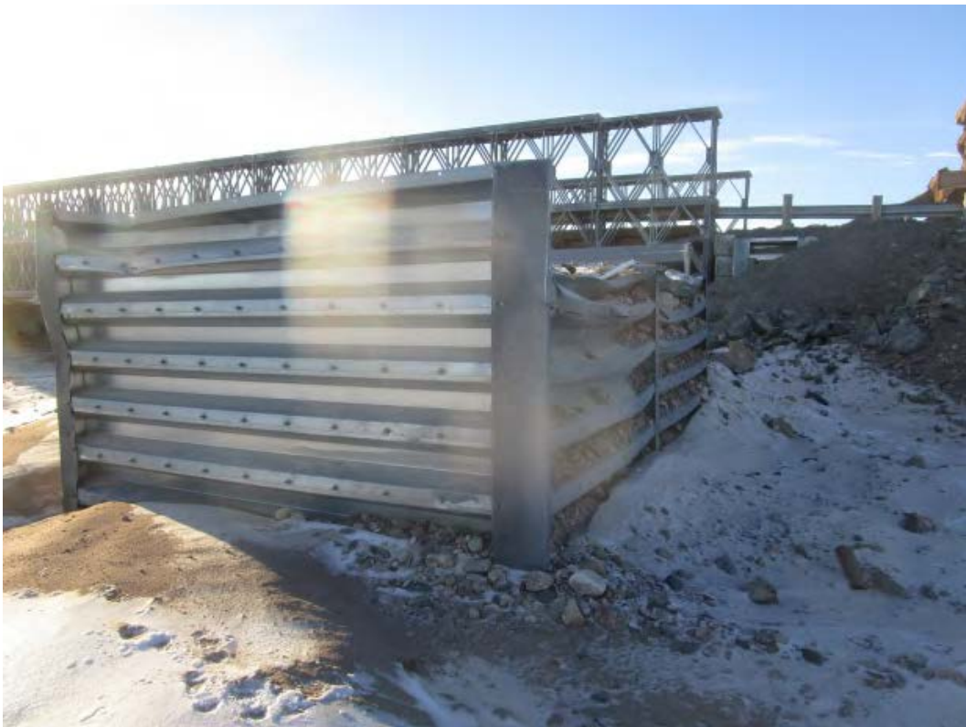
39. Sea can bridge abutments no longer in use. Note there is no deformation.
