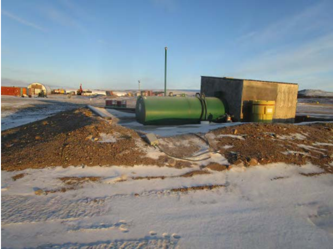
6. Helicopter Fuel Tank Containment.
