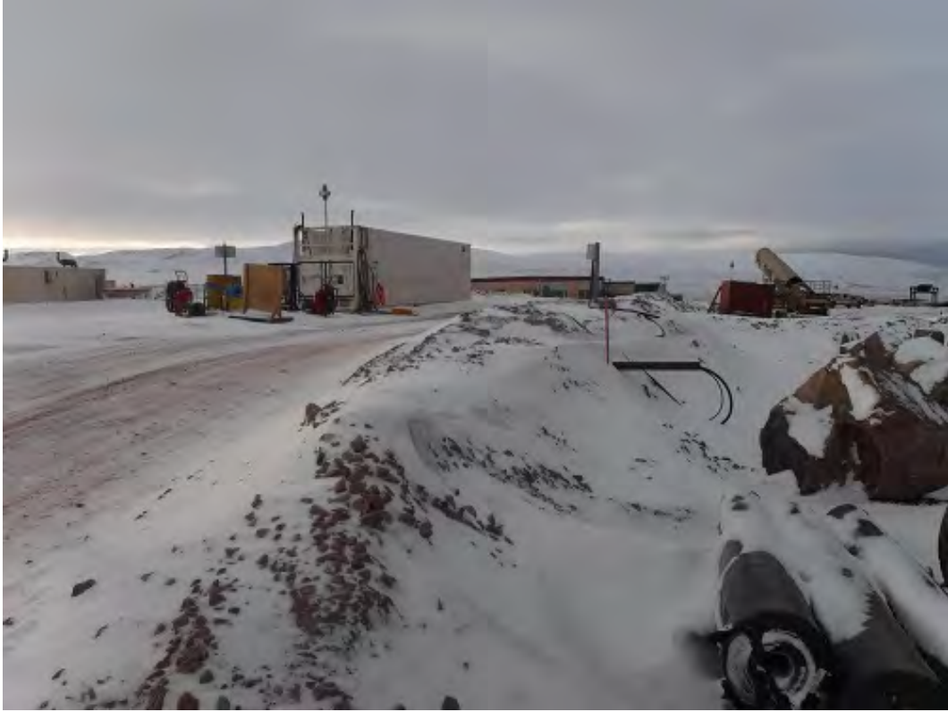
29. Fueling Facility Containment
