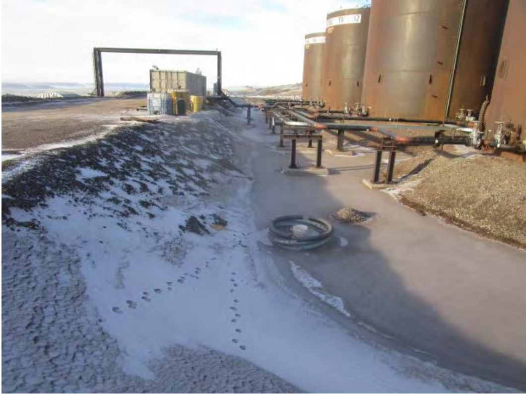
15. Mine Site Steel Fuel Tank Farm Containment.
