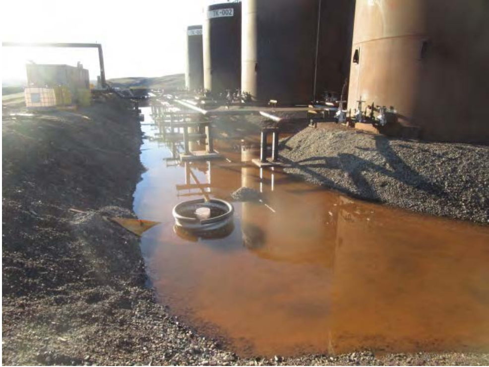
15. Mine Site Steel Fuel Tank Farm Containment
