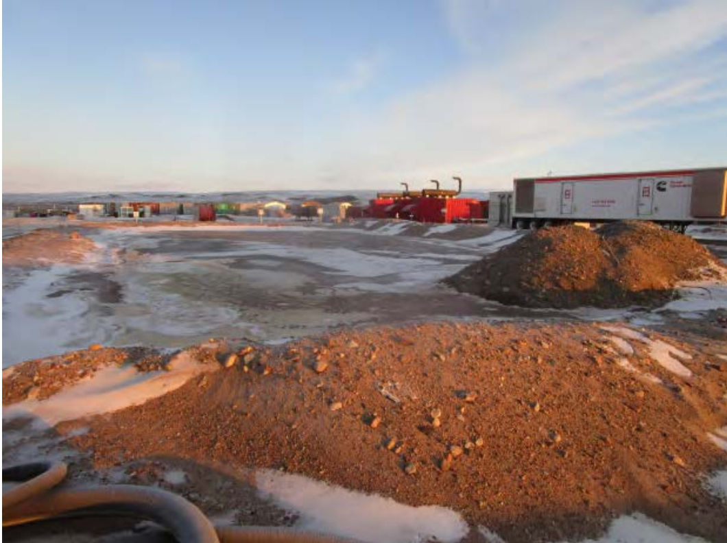
2. Generator Fuel Containment.
