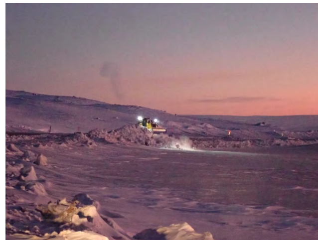
Photo 9-8. Snowbank management (in progress) to facilitate wildlife crossing and improve driver visibility (December 27, 2021).
