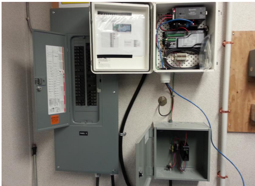
Figure 15: Inside Mary River camp datalogger enclosure and sensor power supply enclosure
