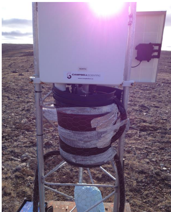
Figure 4: Supplementary chicken wire added to base of Milne station during 2015 maintenance trip
