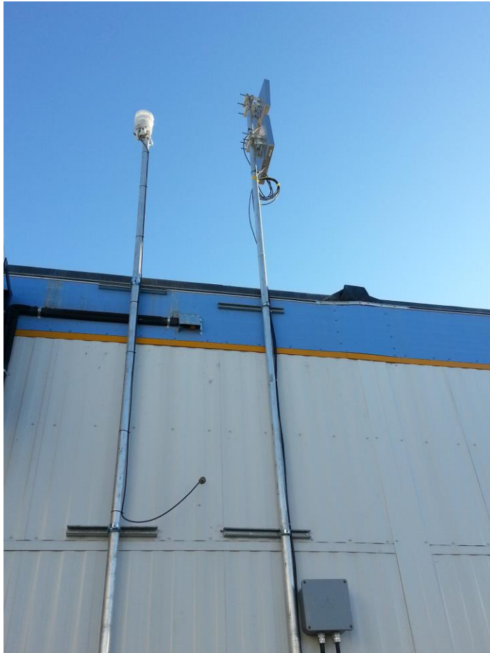
Figure 12: Milne camp WS600-UMB sensor installed on the outside wall of server room trailer (photo taken from 2014 trip)
