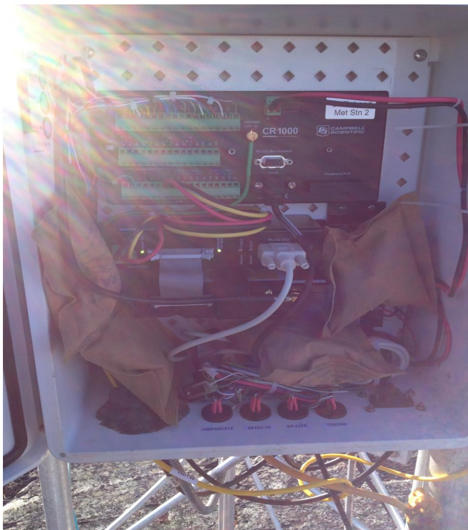
Figure 9: Inside Steensby datalogger enclosure during 2015 maintenance trip
