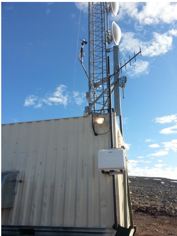
Figure 17: Deposit No. 1 station installed on outside of existing site canister (picture taken during 2014 trip)
