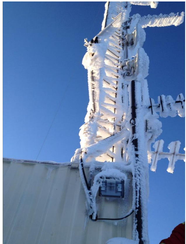
Figure 20: close up of Ice cover on Deposit No.1 sensors during 2015 trip
