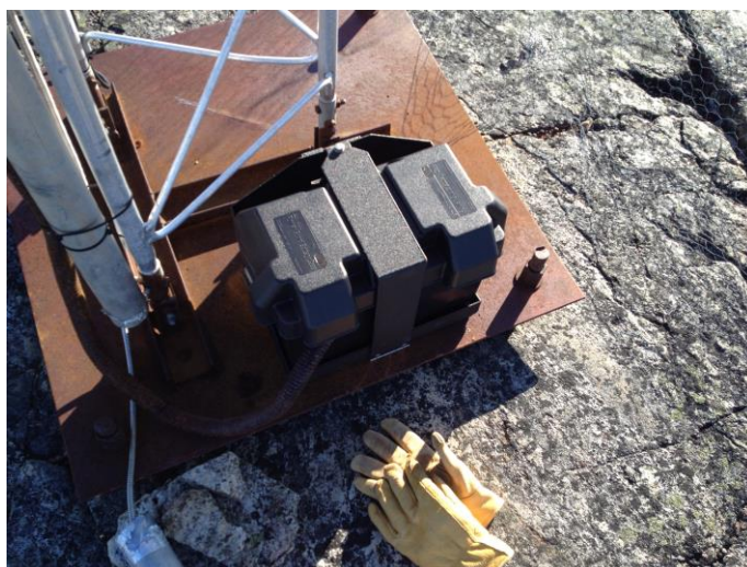
Figure 11: New replacement battery enclosure
