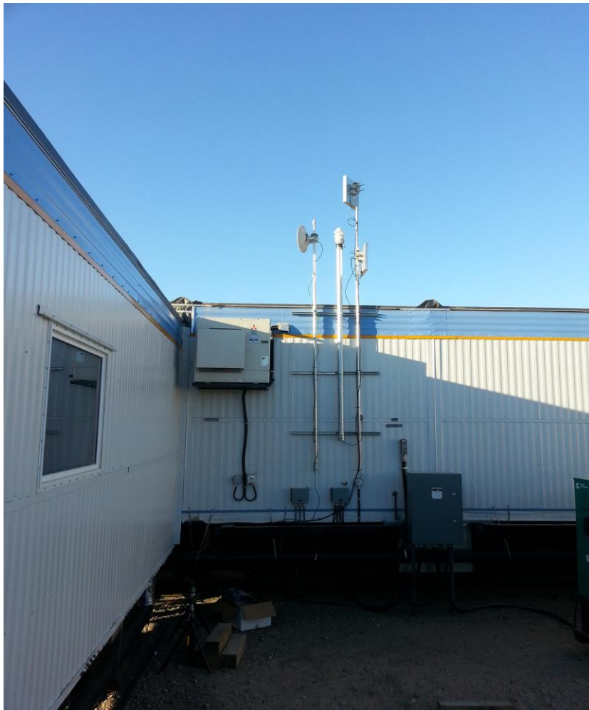
Figure 14: Mary River camp WS600-UMB sensor installed on outside wall of server room trailer (photo taken during 2014 trip)
