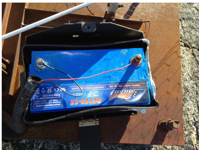
Figure 10: Previous Steensby cracked battery enclosure
