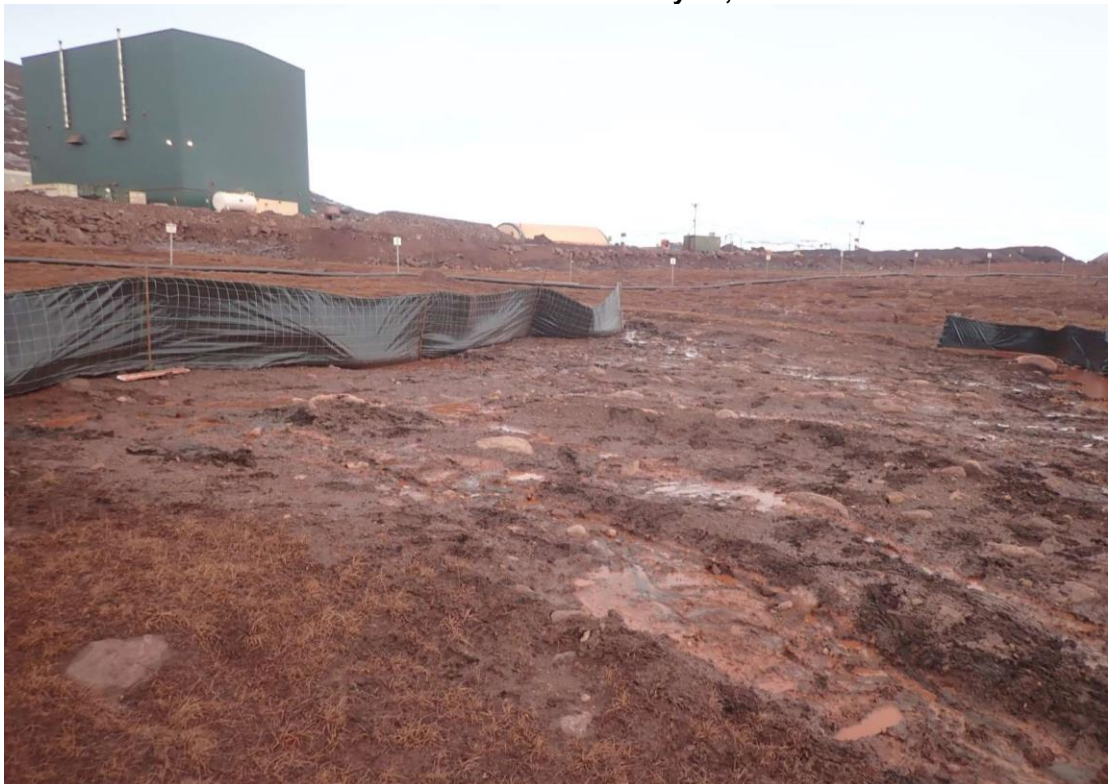
Photo 4. Erosion and Sediment Control Down Slope of Power Generation Building Minimizing Sediment Entering CV-187 (May 22, 2020)
