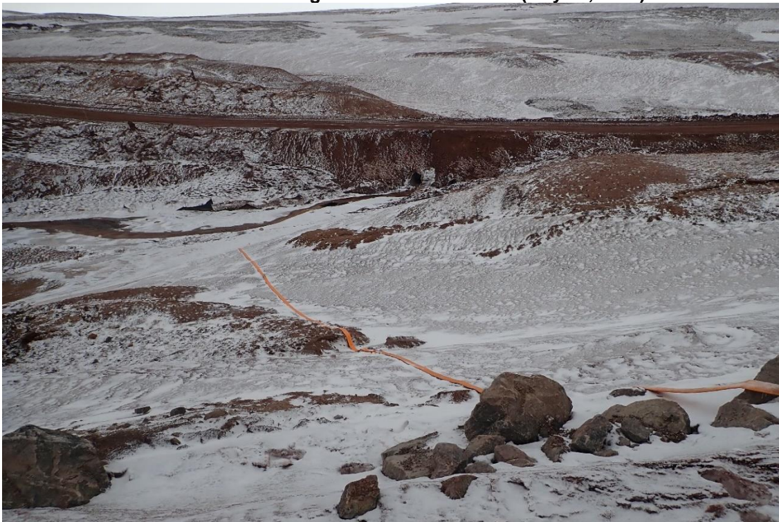
Photo 6. Pumping Diversion from Unstable Sandy Slope at the Outlet of BG-01 (May 18, 2020)
