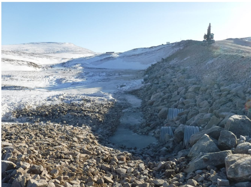
Figure 3. BG01 US installed 17-10-09
