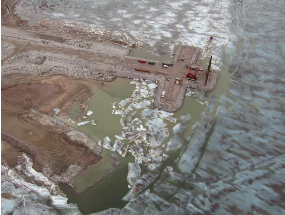
Photo 37 - Aerial view of ongoing construction of the Freight Dock (top) and Barge Lander (bottom), as of 11 June 2019. Photo provided by BIM.
