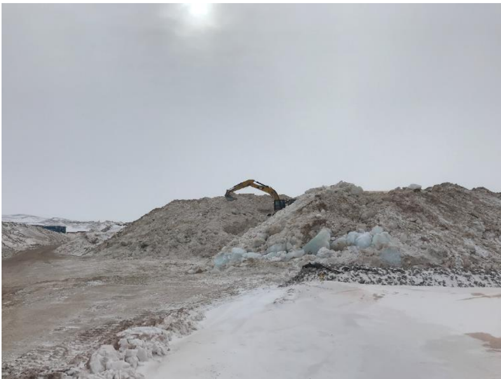
Photo 16 - Snow/sand stockpile extending beyond the containment berm, with excavator working to move material inside the bermed area (looking south), 28 April 2019
