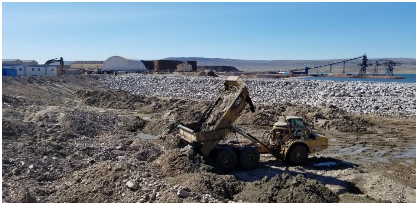
Photo 53 – 45-ton haul truck transporting dredged material to the dredge disposal area, 2 July 2019
