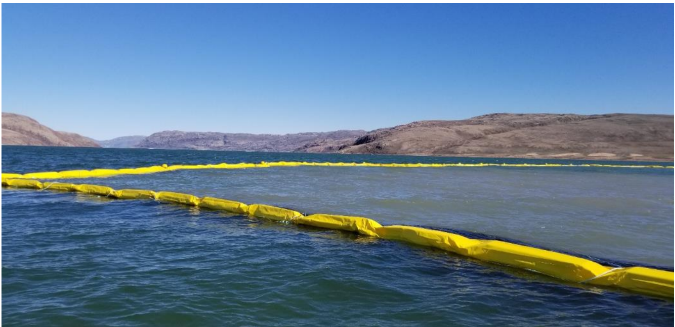
Photo 48 - Silt curtain containing the turbid water within the work area during active dredging, 29 June 2019
