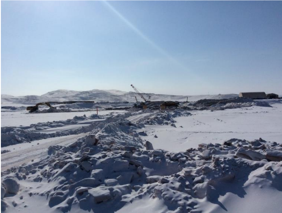
Photo 15 - Placement and compacting of fill material at the Freight Dock causeway, 25 April 2019
