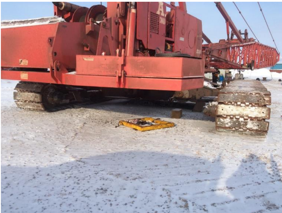
Photo 12 - Secondary containment placed under stationary and inactive crane, 24 April 2019
