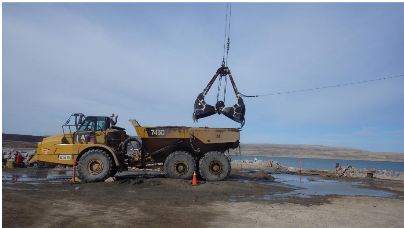
Photo 54 - Loading dredged material into a rock truck for hauling to the dredge material disposal area, 9 July 2019
