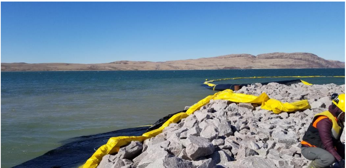
Photo 50 - Billowing panels on the silt curtain releasing plumes of turbid water from the work area, 30 June 2019
