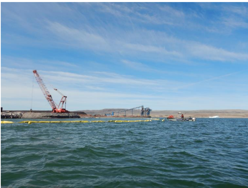
Photo 46 - Nuna deploying panels on the silt curtain prior to dredging activities, 28 June 2019
