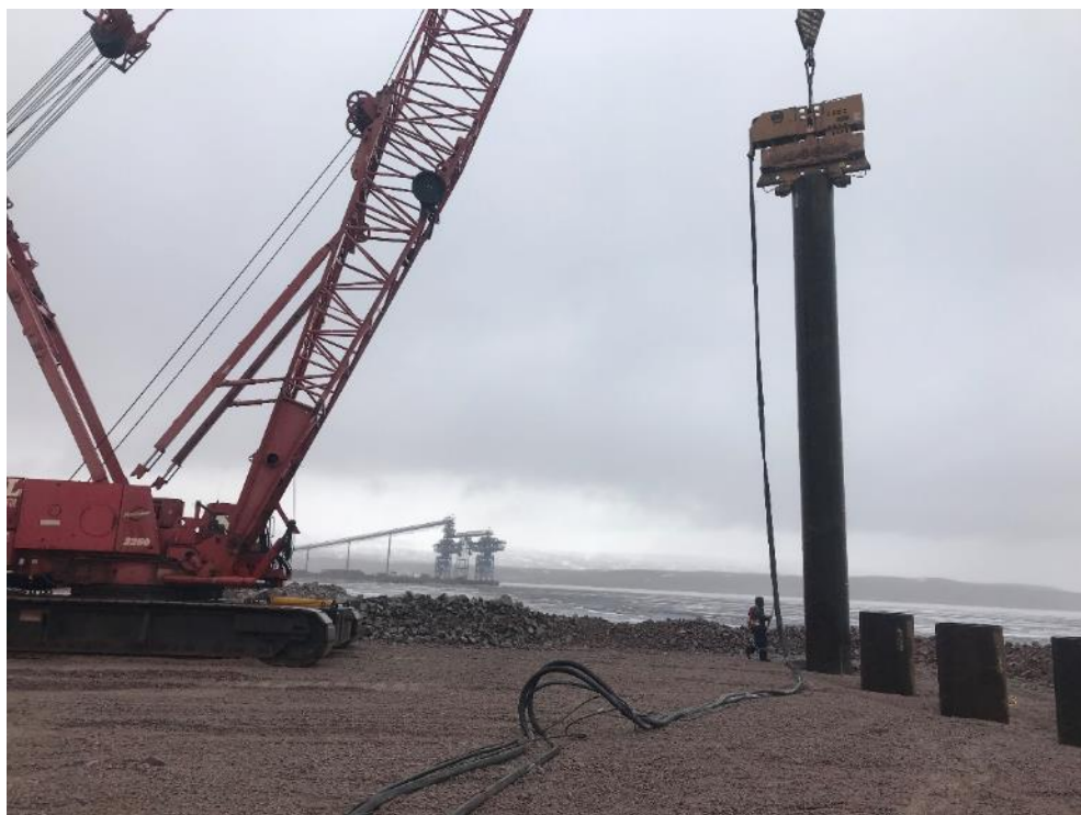
Photo 34 – Vibratory hammering of piles at the north end of the Freight Dock (looking west), 4 June 2019
