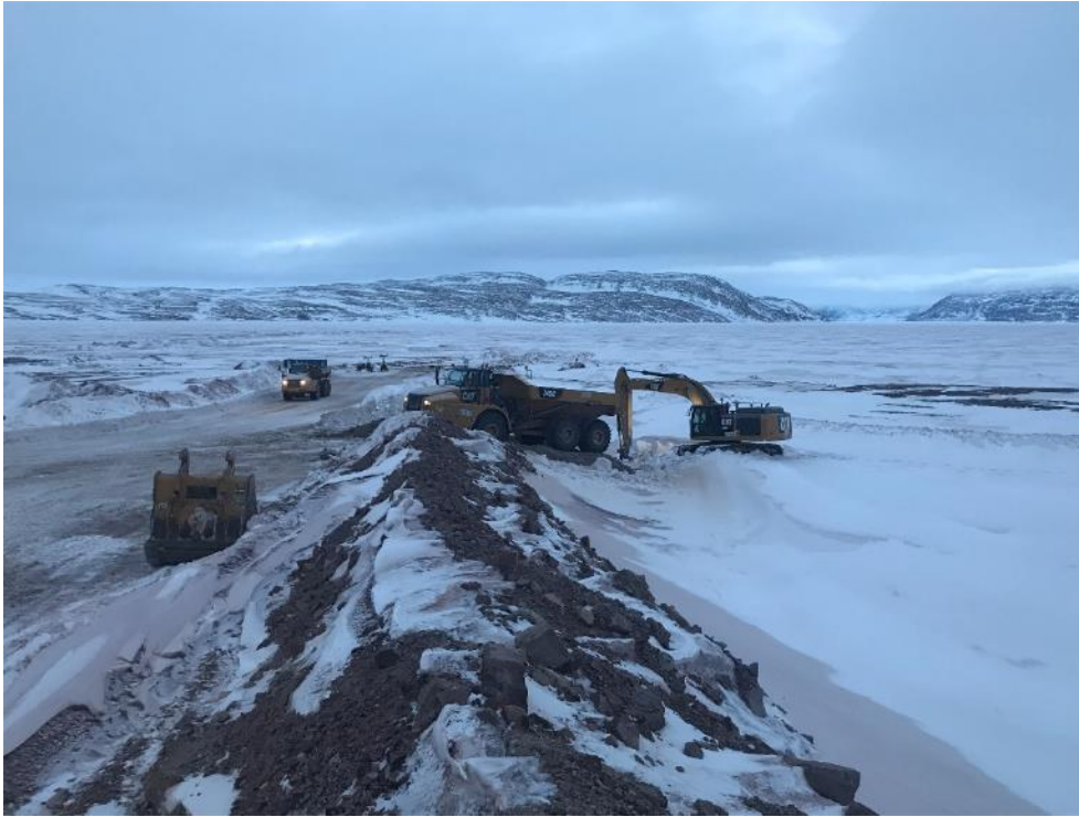
Photo 19 - Vehicle access ramp construction and snow removal at the stream diversion berm area, east of the existing Freight Dock (looking north), 5 May 2019
