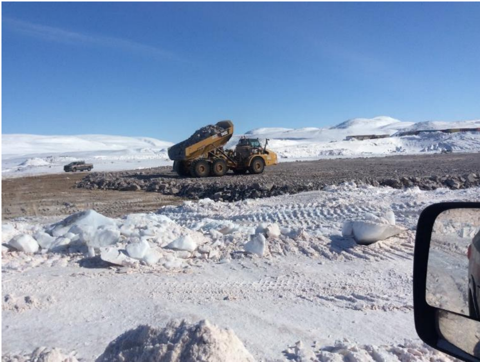
Photo 5 - Placement and compaction of fill material for causeway extension of the proposed Freight Dock (looking south), 23 April 2019
