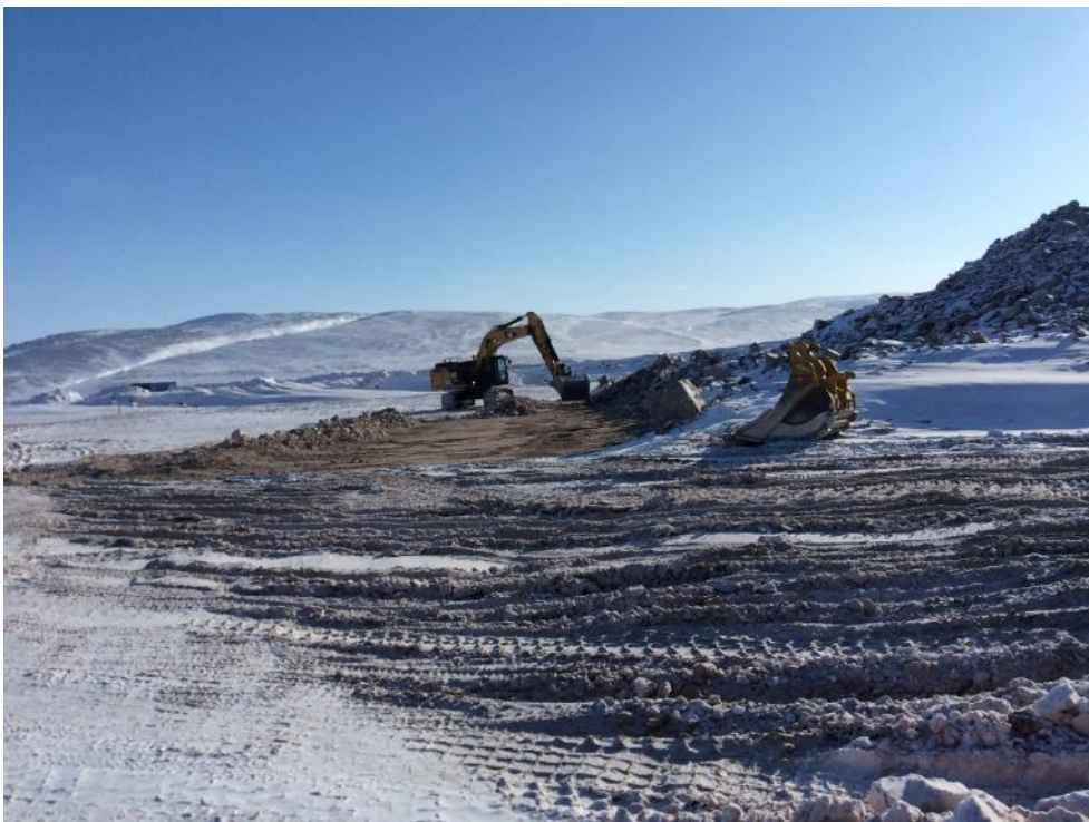
Photo 14 - Snow clearing at the north end of the extent of Freight Dock causeway on 17 April 2019
