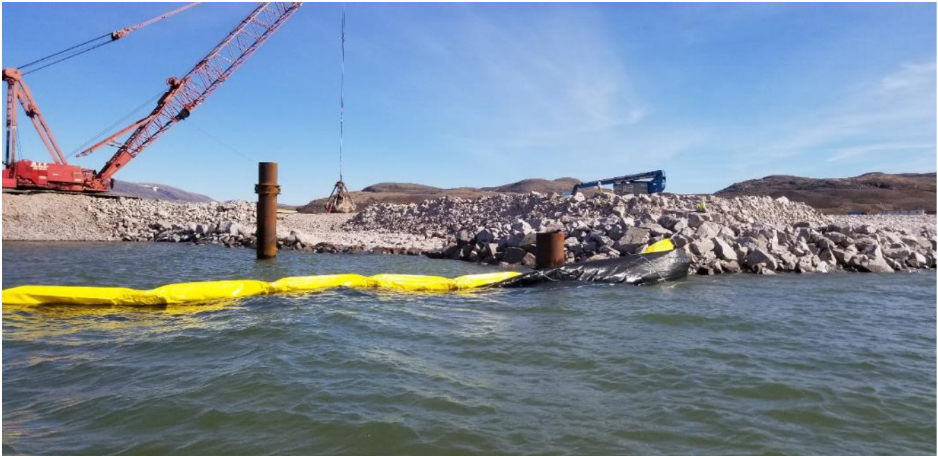
Photo 47 - Falling tide and currents lifting panel on silt curtain off of the west bund on the Freight Dock, 28 June 2019
