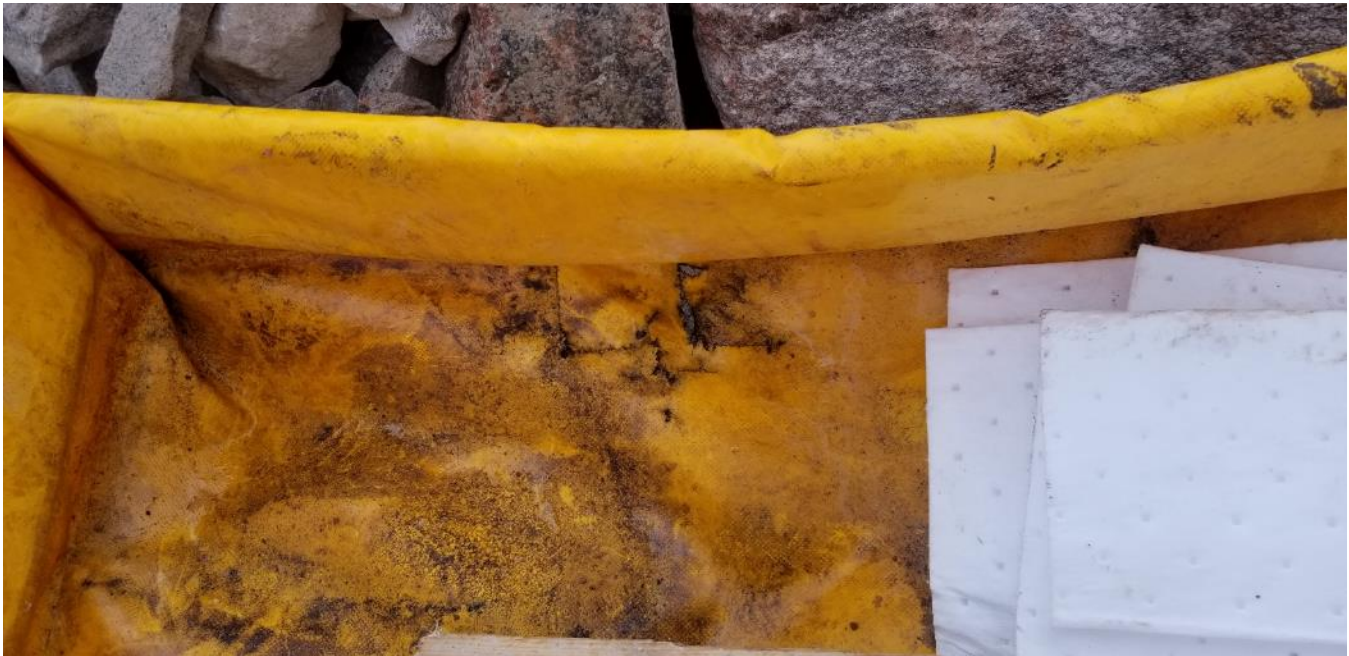
Photo 45 - Tear observed in spill tray located under equipment on the Freight Dock during fueling. A new spill tray was sourced for future fueling, 24 June 2019
