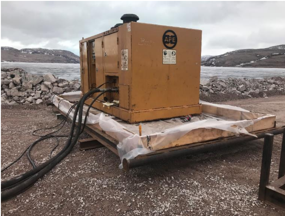
Photo 35 – Vibratory hammer hydraulic power pack in the purpose-built secondary containment (looking east), 4 June 2019
