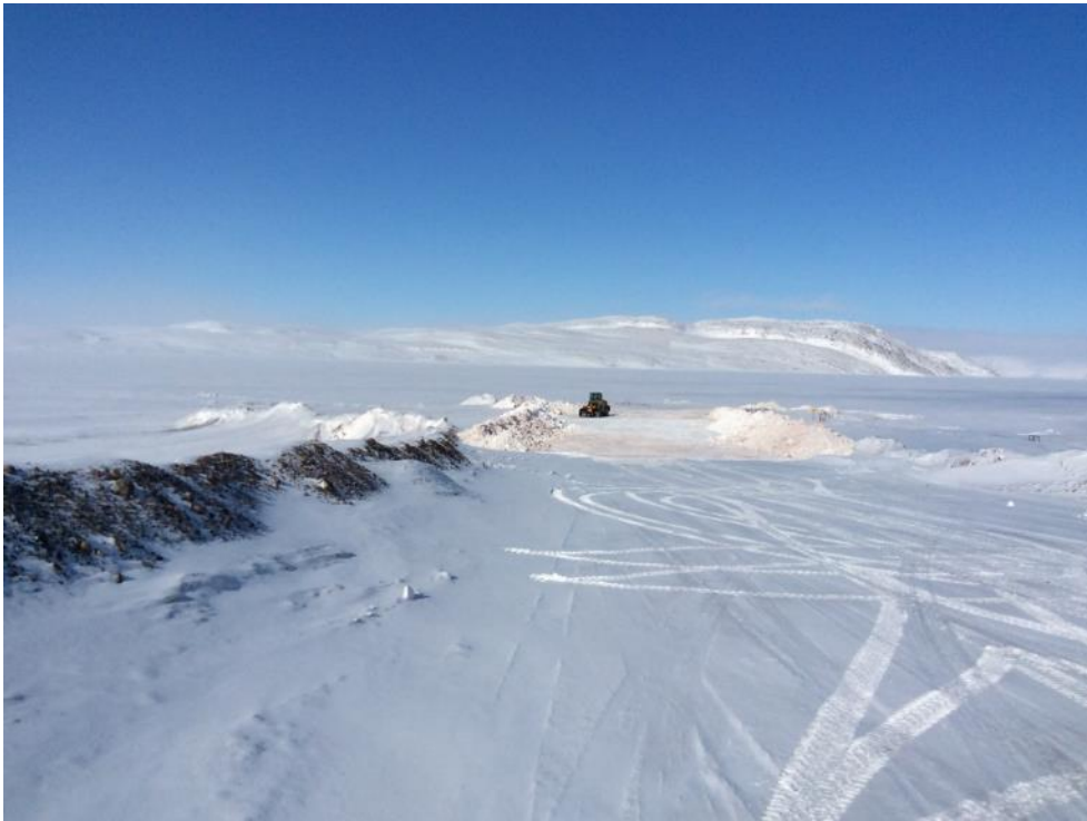
Photo 7 - Snow removal to clear access to existing Freight Dock and ConeTec's laydown area (looking north), 13 April 2019
