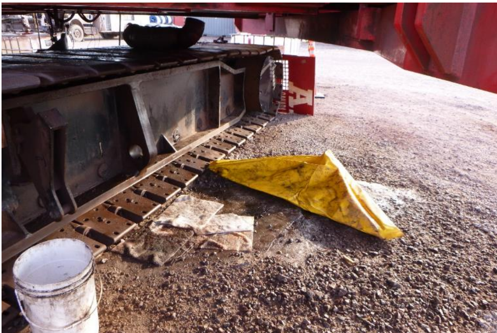
Photo 28 - Previously reported spill left without proper cleanup. Spill tray added to contain further drips was improperly anchored against wind, 22 May 2019
