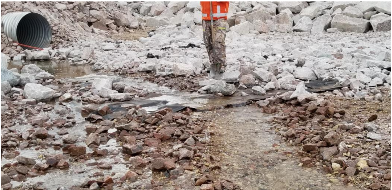
Photo 44 - Restored flow in stream M11-1 following removal of rocks that were blocking fish passage, 24 June 2019
