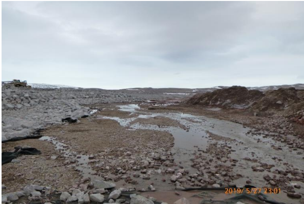
Photo 31 - Stream M11-1, looking downstream from the twin culverts at the old barge lander, 27 May 2019
