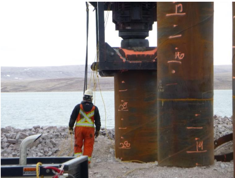
Photo 40 - Diesel hammer performing impact pile driving on pile #1 on the Freight Dock (looking northwest), 17 June 2019
