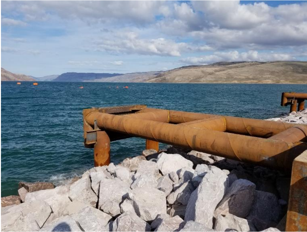
Photo 61 - Looking north from the Freight Dock, following removal of the silt curtain, 10 August 2019
