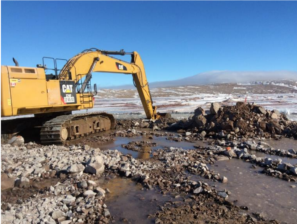
Photo 25 - Excavator dredging at the leading edge of the Freight Dock causeway, 14 May 2019
