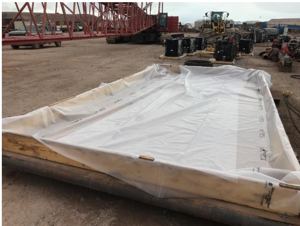
Photo 33 – Custom secondary containment built to contain the vibratory hammer hydraulic powerpack for future work near water, 31 May 2019
