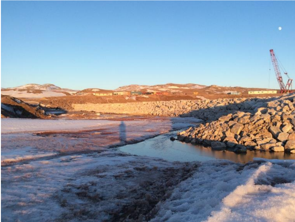
Photo 27 - Completed SWD7 stream diversion berm, with stream M11-1 flowing along planned diverted course, 15 May 2019
