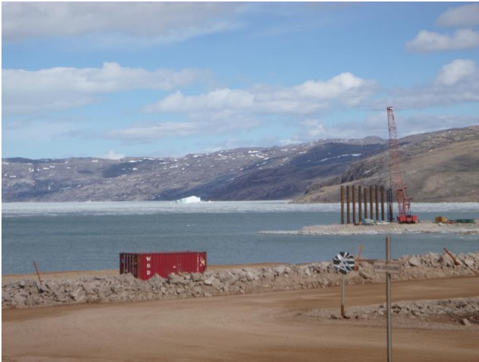
Photo 39 - Sea ice breaking out with southerly wind, during active diesel hammer pile driving (looking north northeast), 16 June 2019
