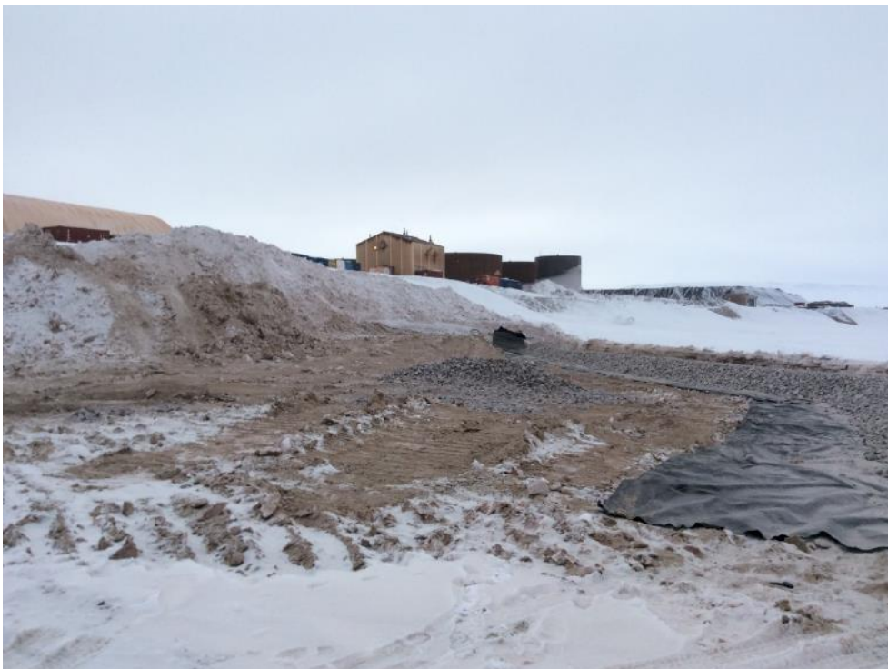
Photo 2 - Filter cloth placement and rock berm for snow/sand containment berm (looking west), 12 April 2019
